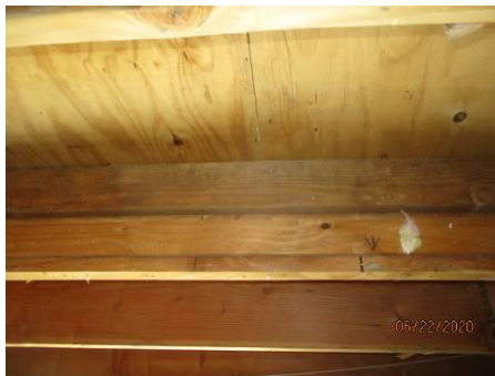
Mold-like growth observed on joist.
