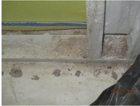
Debris observed on encapsulation.
