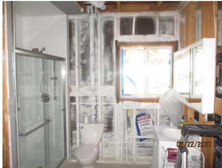
Client stated previous roof leak affected this area.
