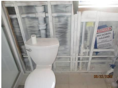
Encapsulation observed on building materials.
