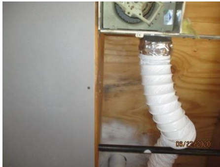
Water staining and discoloration observed on sheathing.
