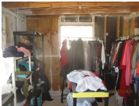
Client stated previous roof leak occurred in area.
