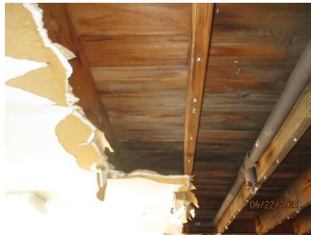
Water staining and discoloration observed on studs, sheathing and joists.
