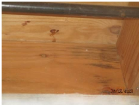
Water staining and discoloration observed on sheathing.
