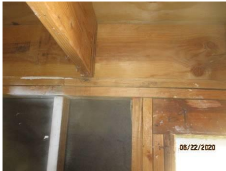
Water staining and discoloration observed on studs.
