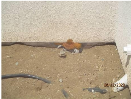
Cracked foundation observed.
