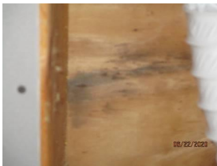
Mold-like growth observed on sheathing.
