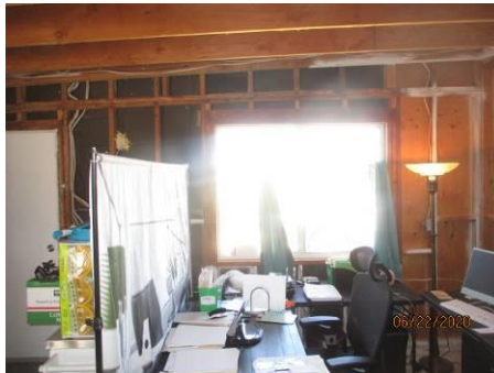
Client stated roof previously blown off and was unmitigated for 40 days.
