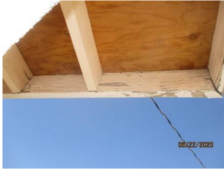
Water damage observed on eaves of roof.
