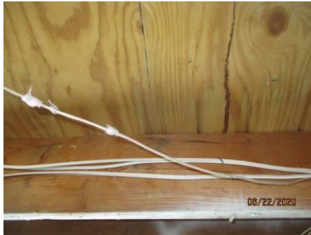
Water staining and discoloration observed on studs and sheathing.
