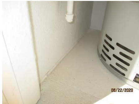
Water staining and discoloration observed around water heater unit.
