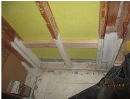
Debris observed on encapsulation.
