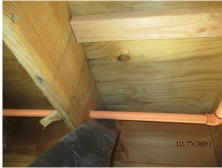
Water staining and discoloration observed on sheathing and joists.
