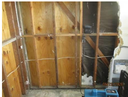
Water staining and discoloration observed on studs, sheathing and joists.
