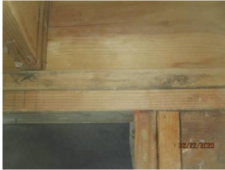
Mold-like growth observed on stud.
