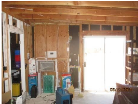
Water staining and discoloration observed on sheathing and joists.
