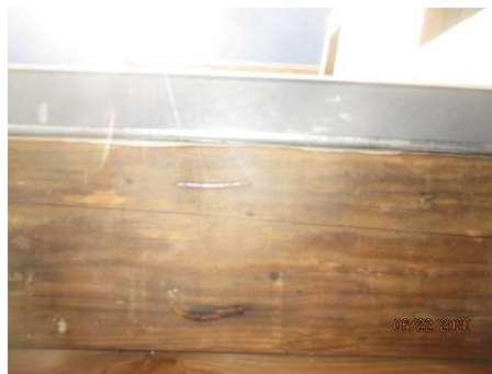
Mold-like growth observed on water heater closet stud.
