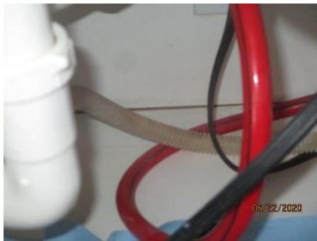
Water staining and discoloration observed under sink cabinetry.
