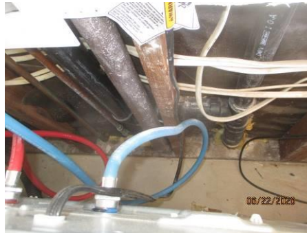
Water staining and discoloration observed on studs and sheathing behind laundry machines.
